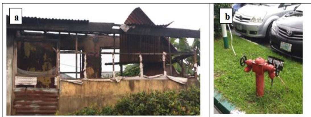
Fig 2a: Fire-ravaged building at number 1, Atekong Street off Big Qua Town hall.
